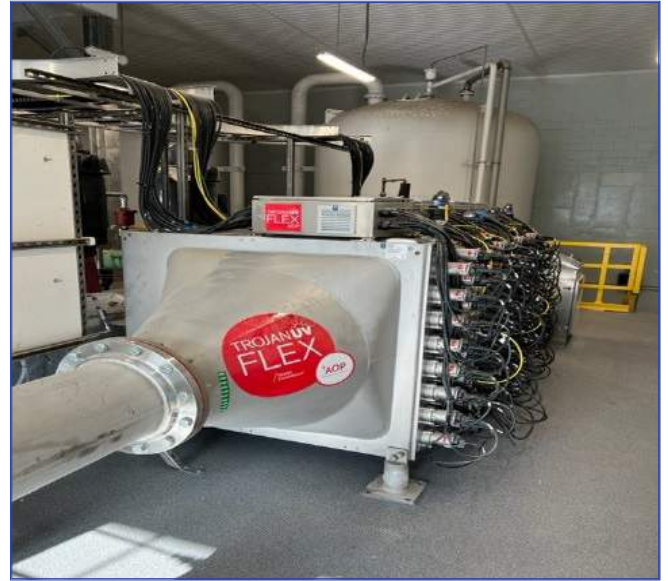
Advanced Oxidation Process (AOP) Treatment System
