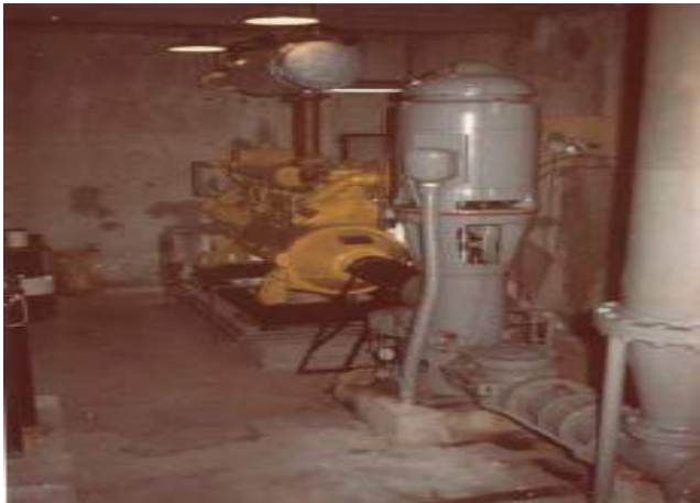
Plant No. 2 Water Supply Well - Circa 1960
