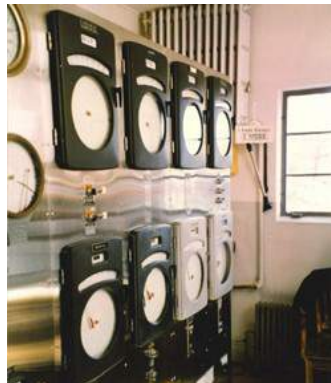
Electrical Telemetry Equipment
