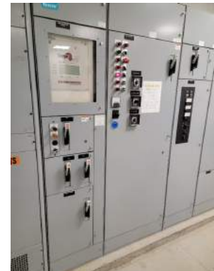
Plant No. 2 Electrical Equipment
