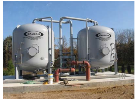
Shutter Lane Granular Activated Carbon Treatment System
